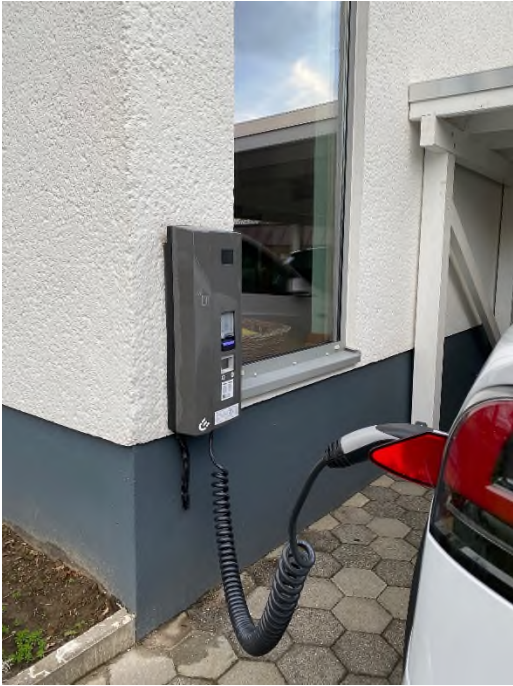
Figure 4: Functional demonstrations for the prototype with a single charging point
